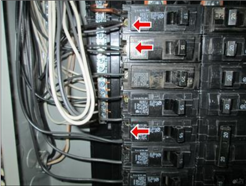
7.1 Picture 1 Right unit Panel
