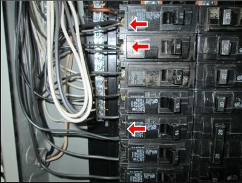
7.1 Picture 1 Right unit Panel
